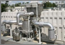
2.35 MW SureSource Hydrogen™ 2.35 MW Power plus 1270 kg/day Hydrogen
