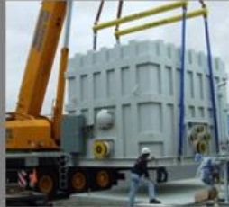
Completed module 1.4 megawatts
